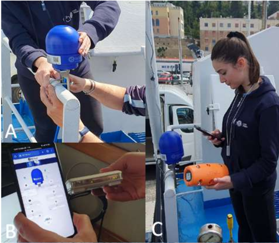
Figure 33: A) WiHub installation operations on board R/V Dallaporta; B) WiHub web interface; C) Setting of the sensor through the web application.
