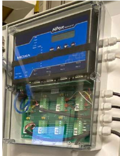
Figure 73: FerryBox serial-to-Ethernet interface junction box with Moxa NPort and serial device connection board.
