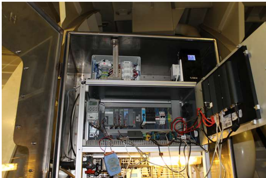
Figure 67. The POSEIDON Ferrybox system power and telemetry module.
