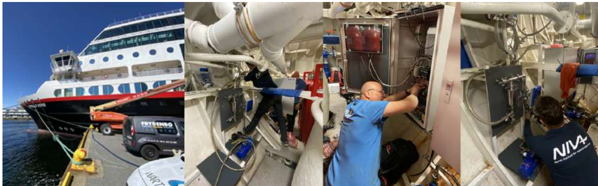
Figure 74: The installation of the microplastic sampling module in the pump room of the Hurtigruten M/S Trollfjord.
