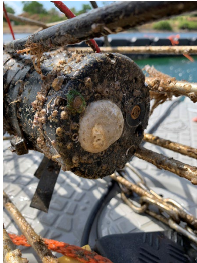
Figure 17: Development of an unexpected chemical reaction on the surface of the detection cell damaging the silicate sensor after a few days of field validation
